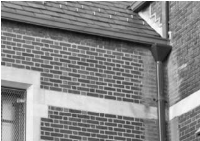
▲ Undersized gutters led to facade deterioration at eaves and downspouts.
