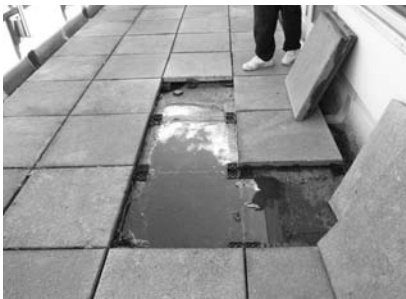
▲ At the surface, these pavers seem fine. But trapped water below may be causing leaks.
