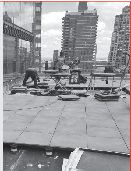
▲ Installation of a roof terrace with bituminous waterproofing membrane, board insulation, and pavers-on-pedestals.
