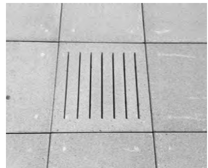
▲ Slotted pavers over drains provide a clean look and even surface.
