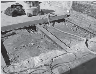
▲ To support the added load of plantings and pedestrians, existing structural framing may need to be exposed and augmented.
