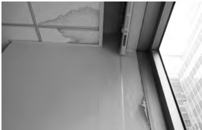
▲ Leaks and drafts.
