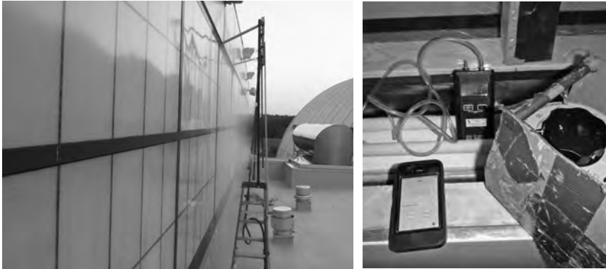
▲ Field water penetration test to investigate leaks at an existing glazed curtain wall assembly.
