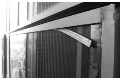
▲ Failed gaskets and seals.
