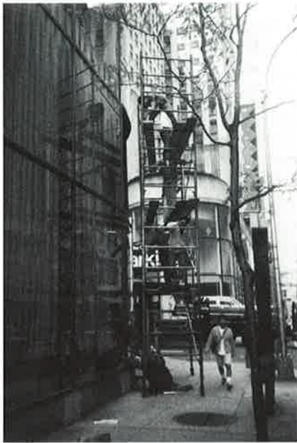
Investigation of leaks in a bronze-and-glass curtain wall on a New York City building.
