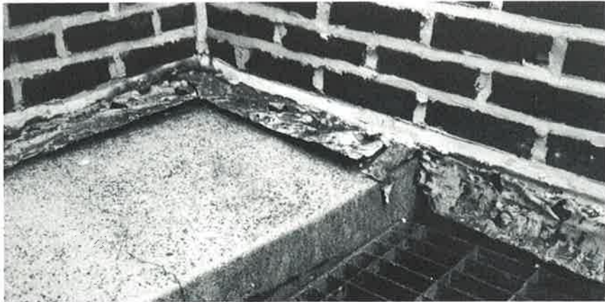
This completely deteriorated copper counterflashing was not replaced when the wall was re-pointed, a poor effort in itself.
