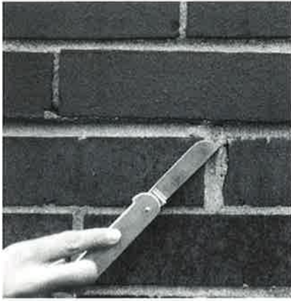
A rather poorly constructed masonry wall. Note the many openings in the mortar, which allow water entry.
