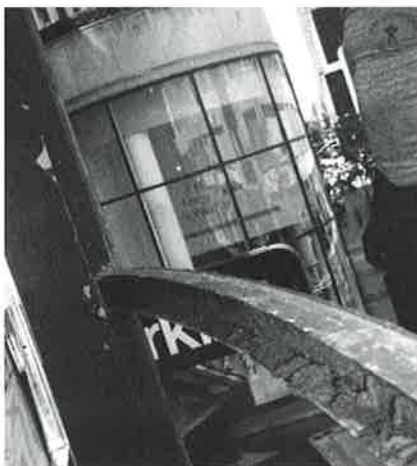
Rust has formed on the steel supportive structure behind this leaking bronze-and-glass curtain wall.
