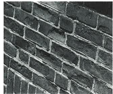
The brick has lost its face from water entering the wall through the back of the parapet.
