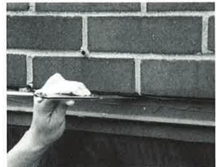
Adhesive failure of the sealant at the joint connecting the brick masonry, wall flashing, and aluminum window.
