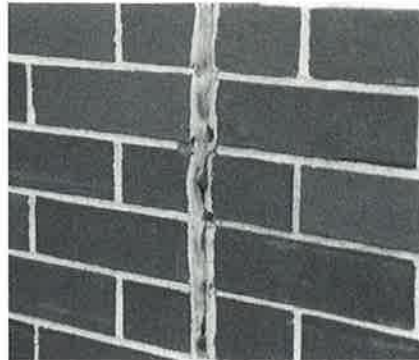
Cohesive failure of the sealant in a brick masonry expansion joint.
