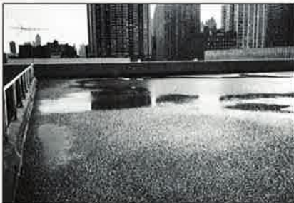
Standing water – a sure sign of insufficient slope for proper drainage.
