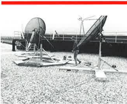
Large support bases for satellite dishes evenly distribute imposed loads.
