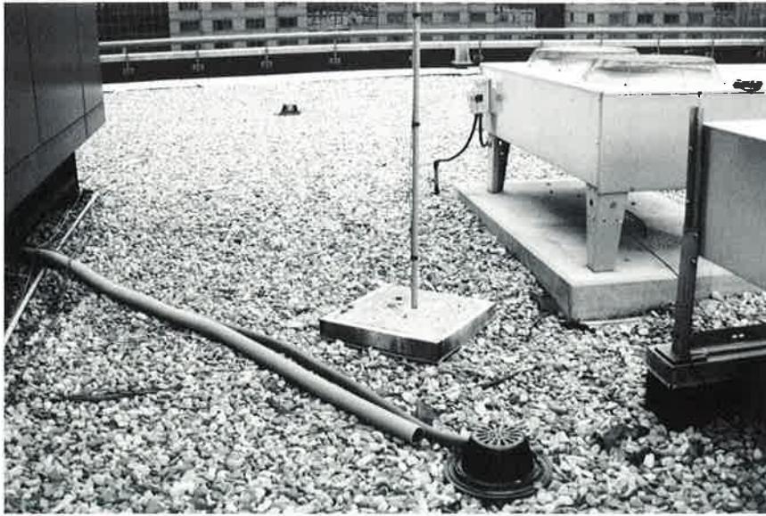
Poured concrete support pads are improperly placed directly on stone ballast.
