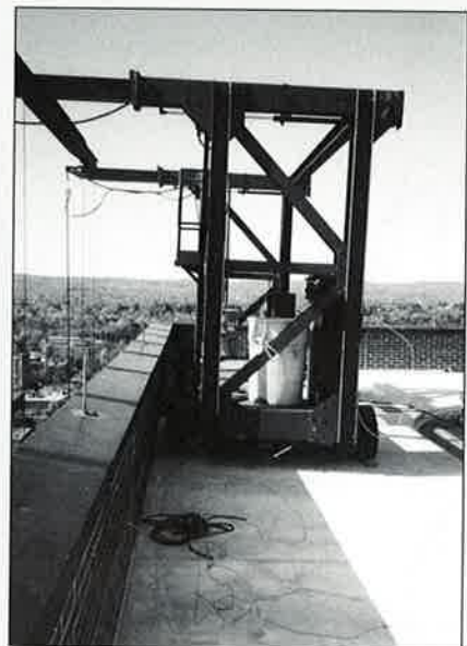
Poured-in-place concrete runway acts as a wearing surface and distributes the weight of the window washing rig carriage.
