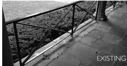
▲ Railings at historic terrace are too low, with openings that are too large.
