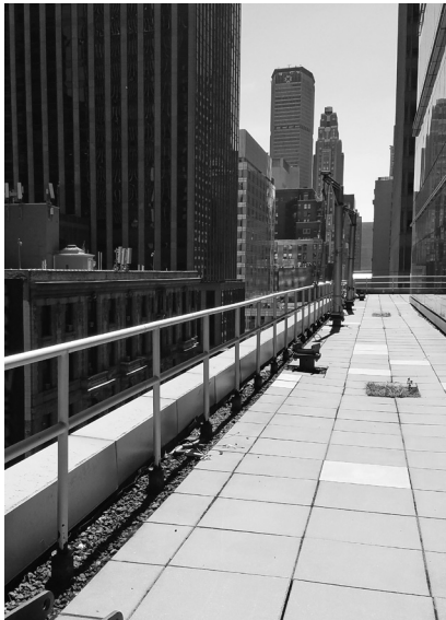
▲ As codes change, owners may find that existing railings must be updated or replaced.
