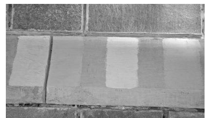
▲ Field testing of coating samples for best match to original color and gloss.
