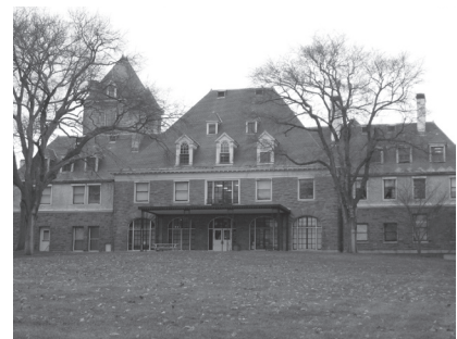
▲ Fairfield University, McAuliffe Hall (pictured), and Bellarmine Hall in Fairfield, Connecticut. Slate Roof and Building Envelope Rehabilitation
