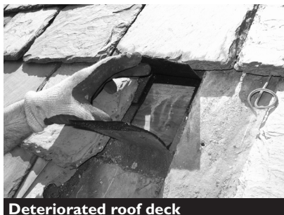
Deteriorated roof deck
