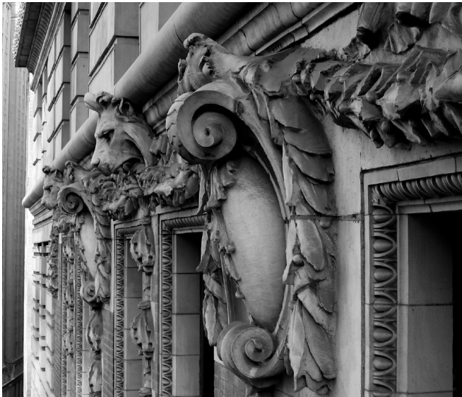
▲ Often finished in imitation of stone, terra cotta can be difficult to recognize and may be mistaken for cast stone, concrete, stone, or brick.
