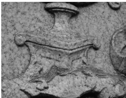
▲ Failed prior repair effort.
