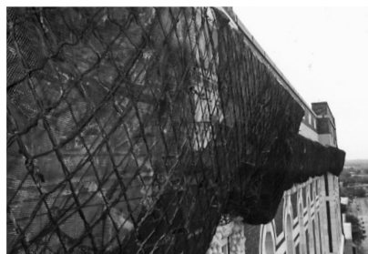
▲ Until permanent repairs are made, netting may be used to secure unstable terra cotta.
