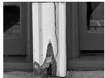
▲ Crack and spall caused by corroded steel.
