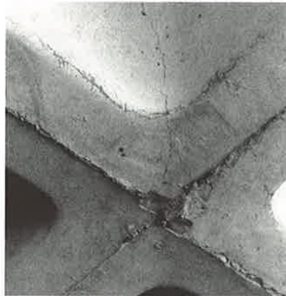
cracking in a waffle slab
