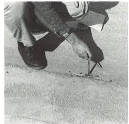
deterioration of joint sealant
