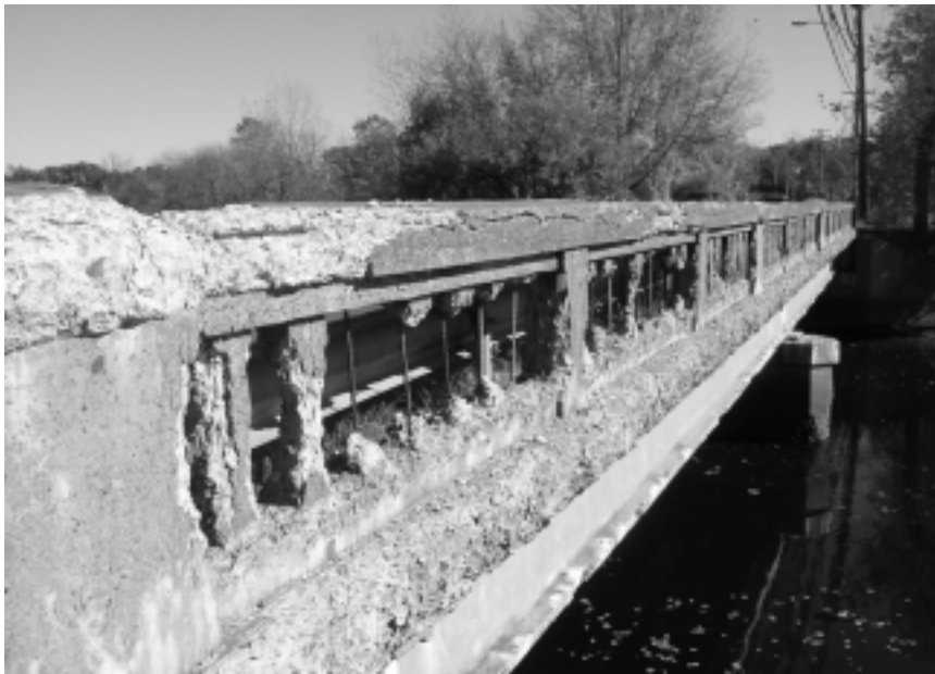
A concrete bridge parapet wall exhibits severe deterioration caused by repeated freezing and thawing cycles.
