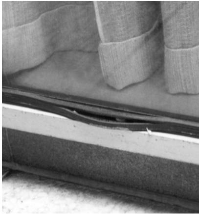
A Figure 3. Failed gasket at the base of the glazed curtain wall will permit water and air penetration.
