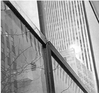
A Figure 4. The metal support system behind the mullion cover has rusted, causing it to extrude.
