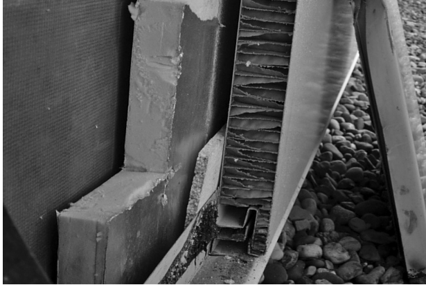
A Installed in the 1990s, this metal cladding system consists of painted steel composite panels with a paper honeycomb core. Rigid insulation, inboard of the panels, provides thermal resistance.
