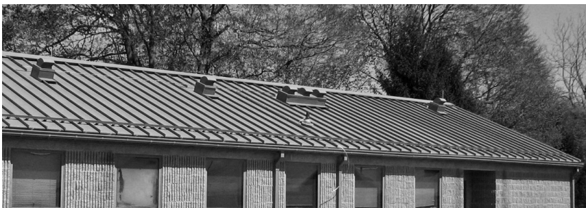
▲ For this military training camp, standing-seam aluminum roofs with a high-performance resin coating met fast-track project demands, while offering durability in the harsh seaside climate.
