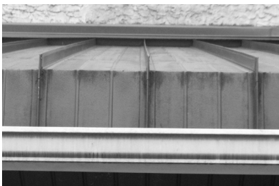
▲ Discoloration and staining
