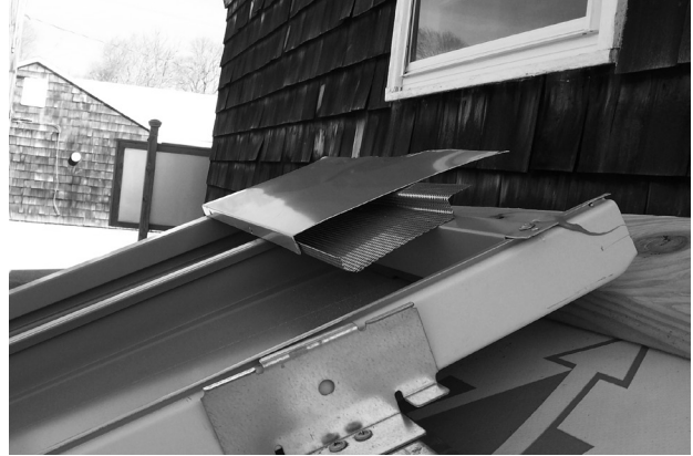
A This aluminum standing-seam roof system is installed over ice dam membrane, as well as stiffening ribs at the flat of each panel to minimize oil canning and telegraphing of structural members.
