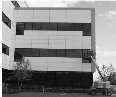
▲ Leak investigation at this steel panel facade pointed to faulty installation practices.
