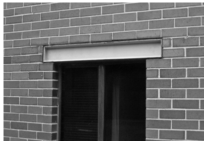
▲ This steel lintel acts as a thermal bridge, conducting heat through the building exterior.
