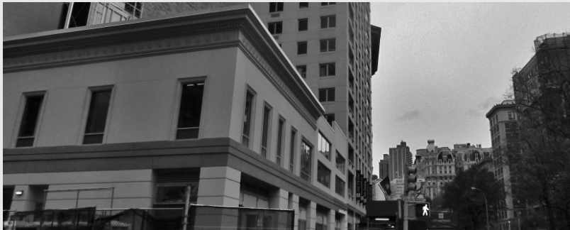
▲ Overcladding of an existing brick masonry building with exterior insulation and finish system (EIFS).
