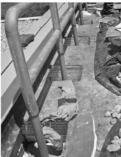
▲ Considerations for railing installation at this roof include thermal bridging and achieving correct railing height due to added insulation.
