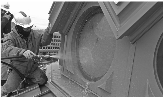
▲ Static and dynamic water penetration tests confirm the window assembly's conformance with design specifications.
