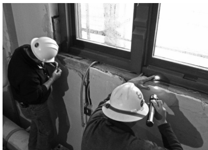
▲ Water infiltration field testing involves close analysis of frames and wall openings.
