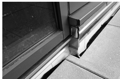
▲ Where roof, window, and wall systems interface, custom details may be necessary.
