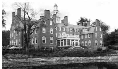
Choate Rosemary Hall, Archbold Building in Wallingford, Connecticut. Window Replacements and Exterior Upgrades.
