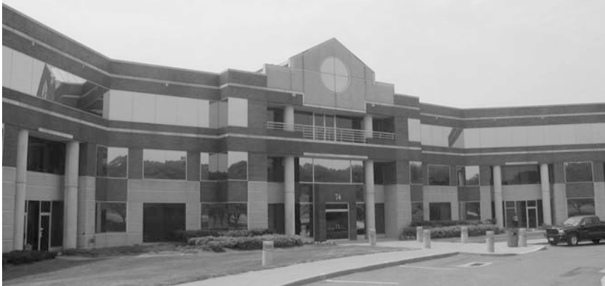
▲ Pond View Corporate Center Farmington, Connecticut. Hoffmann Architects conducted a water infiltration investigation of the facade and developed a program to rehabilitate this corporate facility.
