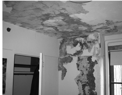
▲ Interior finish damage from roof leaks.
