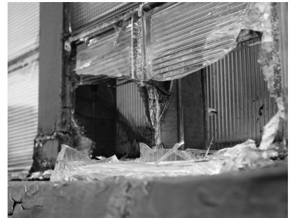
▲ Shattered glass block windows.
