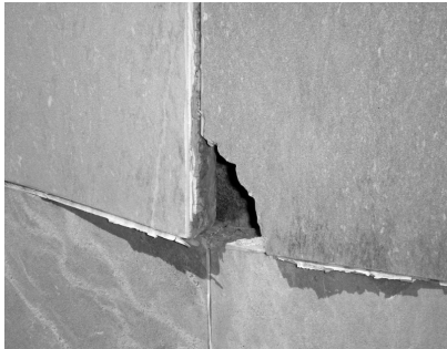
▲ Displacement and fracture at stone facade.
