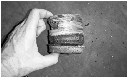
▲ Test cores may be used to evaluate conditions within a roof assembly.
