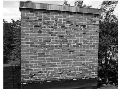
▲ Spalled brick masonry at chimney.
