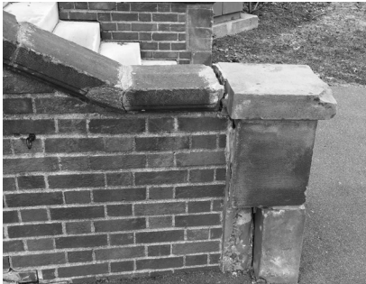
▲ Site wall and exterior stair damage.
