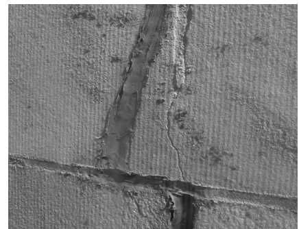
▲ Incorrect use of sealant.
