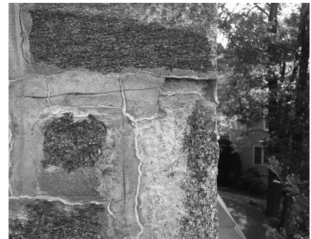
▲ Deteriorated face-pointed mortar.
