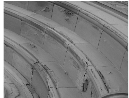
▲ Blistering waterproof coating.
