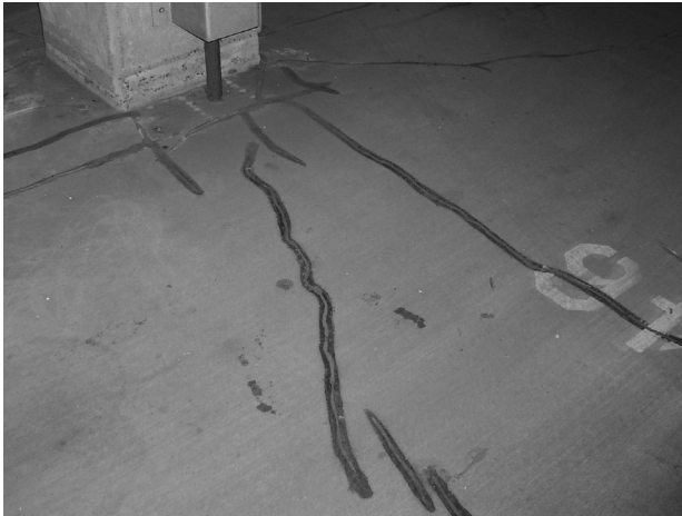
A Cracks are routed and sealed before application of a penetrating sealer.
