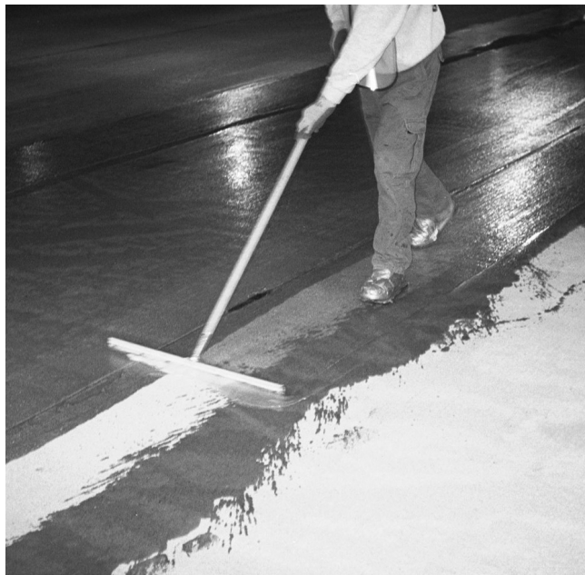
▲ Applying a low-cost sealer to a concrete deck can be a quick, effective, low-maintenance option.
