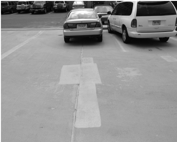
A Edges of pre-cast concrete units at sealant joints catch snow-plow tips, quickly wearing away surface treatments. Here, coating patches were used as a temporary fix.
