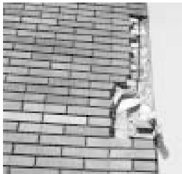
▲ Restricted movement at a joint prevented expansion of this masonry tile, which then broke under the pressure.
