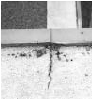
▲ Differential movement of the steel and foam on this roof has led to severe cracking. Like wood, foam also expands and contracts with moisture, further exacerbating the damage.
