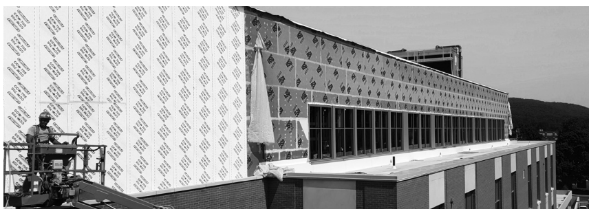
▲ At the top level of this energy-efficient building, an adhered air barrier provides the primary weather protection for a metal panel cladding system, to be installed.
