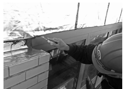
▲ A technician repairs a penetration in an air and vapor barrier system.
