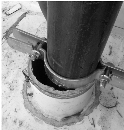
▲ An open pipe penetration spotted during a waterproofing consultation.
