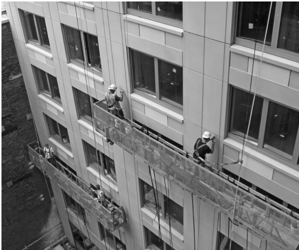
▲ Technical details, such as sealant joint design, make the difference between a long-lasting building and one that fails prematurely.
