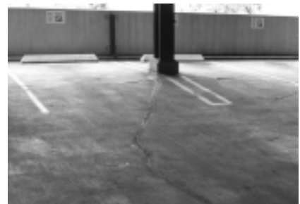
▲ Cracks and settlement of concrete slab.
