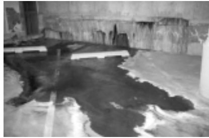
▲ Obvious indicators of water infiltration are ponding and staining.
