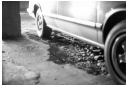
▲ Crumbling parking deck.
