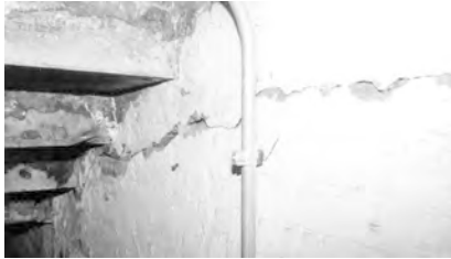
▲ Cracking and spalling in interior spaces below a plaza is an indication of water infiltration.
