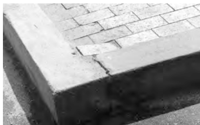
▲ Cracks and heaved pavers, tripping hazards, are among the indicators of failure in plazas.
