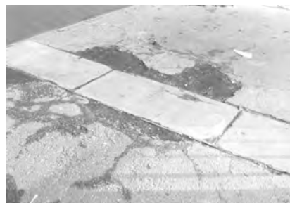
▲ Evidence of deterioration in plazas is commonly apparent as water stains, cracks and spalls. The poured plaza wearing surface above exhibits all of these.
