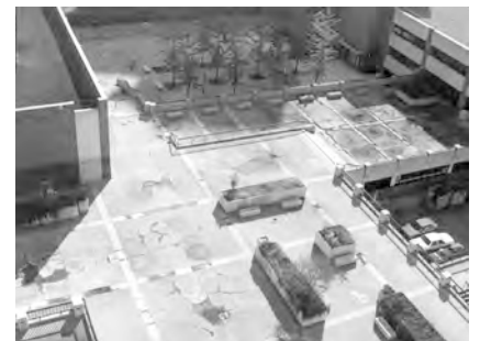
▲ Pro-active repairs and maintenance measures could have prevented the many failures at this plaza.
