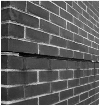
▲ Corrosion of steel shelf angle.
