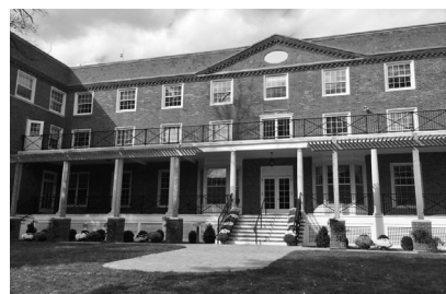
▲ Chase Collegiate School, Saint Margaret's Hall in Waterbury, Connecticut. Portico and Masonry Rehabilitation.
