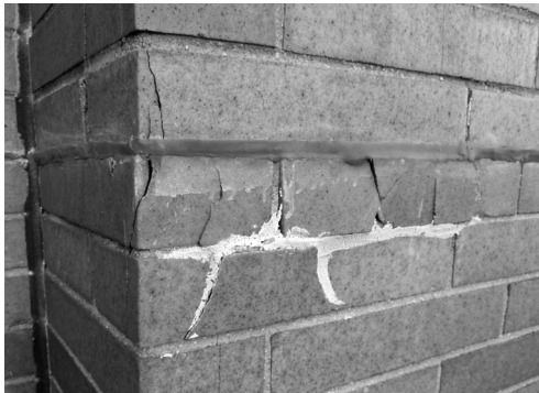
▲ Sealant alone cannot resolve masonry distress.
