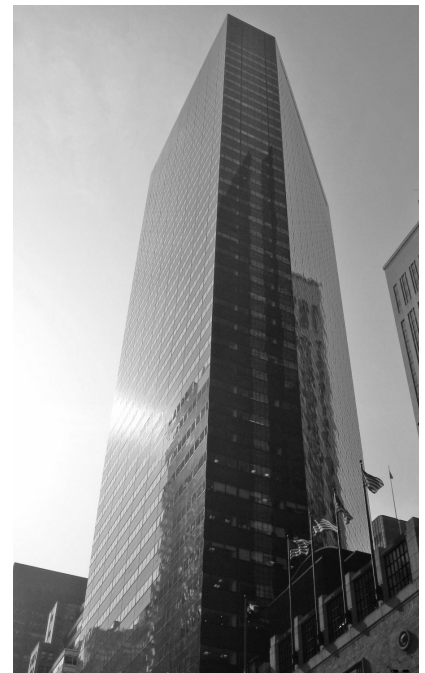
▲ Edward J. Minskoff Equities at 590 Madison Avenue in New York, New York. Glass/Granite Curtain Wall Repair.
