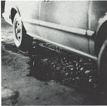
concrete deterioration in parking garage
