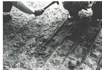
testing adhesion of deteriorated concrete to reinforcing bars
