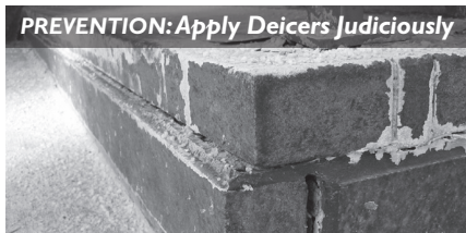
Corrosion and Deterioration
