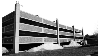
▲ Lahey Clinic Hospital in Burlington, Massachusetts. Parking Garage Investigation and Weather Damage Rehabilitation.
