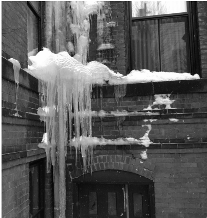
▲ Icicles might seem like charming seasonal decorations, but they mean trouble – both for the building and for those below.
