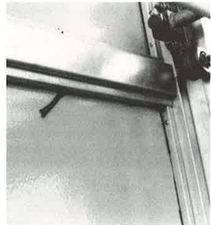
failed sealant in aluminum curtain wall
