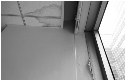
▲ Leaks and drafts.
