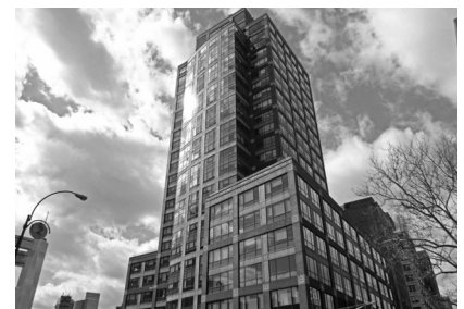
▲ 101 Avenue of the Americas, New York, NY, Modified Bitumen Roof Condition Survey.
