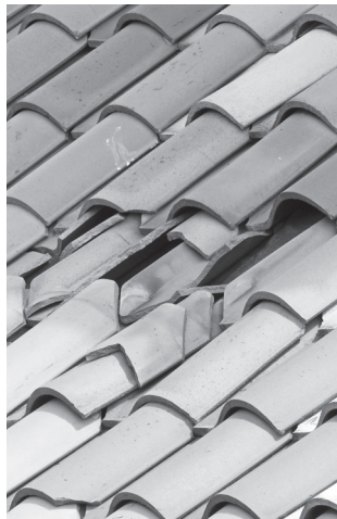
▲ Broken tiles or shingles.
