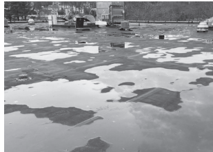
A Ponded water.
