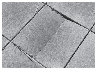
A Cracked pavers.
