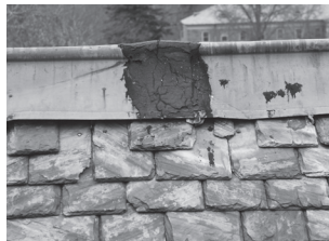
▲ Failed past repairs.
