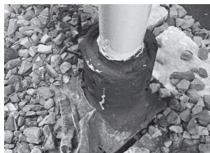
A Damage at roof penetrations.
