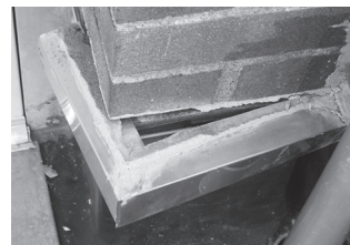
A Displaced / damaged flashings.
