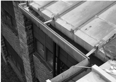
▲ Clogged with debris, these inadequate gutters are filled with standing water.
