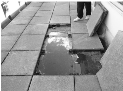
▲ At the surface, these pavers seem fine. But trapped water below may be causing leaks.
