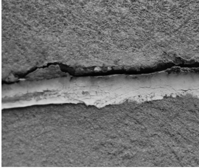
▲ Adhesive failure: Sealant pulls away from the substrate.
