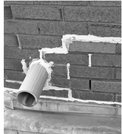
▲ Sealant misused to repair mortar joints.
