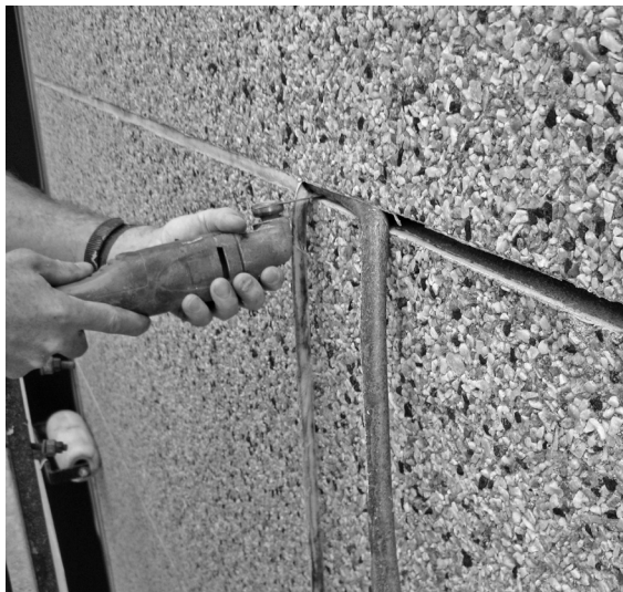
▲ Facade sealant replacement begins with complete removal of existing sealant and backer rod.
