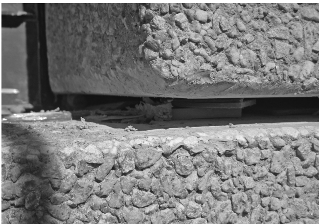
A Insufficient joint preparation can compromise sealant adhesion. Debris and residue must be cleaned prior to new sealant installation.
