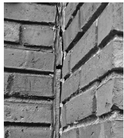
▲ Failure to maintain sealant joints can lead to severe deterioration and water entry.
