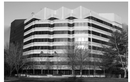
▲ Vornado/Charles E. Smith, Crystal City Office Complexes in Arlington, Virginia. Sealant Remediation at Eleven Buildings.
