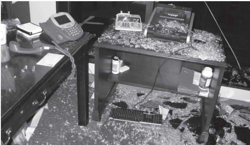
▲ Even a small breach in the building envelope can lead to serious devastation as tremendous wind pressures build inside the structure.
