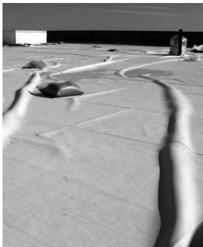
A Sandbags temporarily secure this roof membrane, which detached during a storm.
