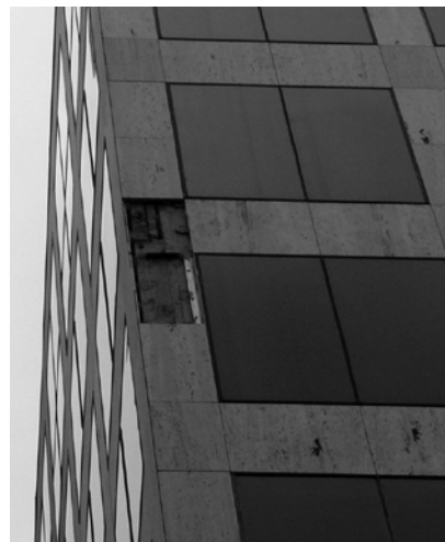
A Insufficient anchorage allowed this stone panel to blow off in a hurricane.
