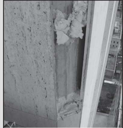
A Insufficient load capacity compromised the wind resistance of these panels, which otherwise might have remained intact.
