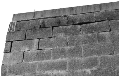
▲ Failure investigation, remediation, and litigation support at a state facility.
