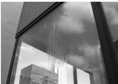
▲ Condensation doesn't just cloud the view, it points to poor thermal performance.
