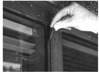
▲ Failed sealant provides a pathway for heat, air, and moisture transfer.
