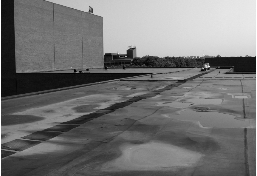
▲ Inappropriate materials selection can mean early replacement—and wasted resources. When wind pressures proved too great for the self-adhered insulation on this roof, the material pulled apart and shifted under the membrane.
