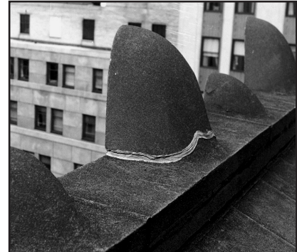
▲ Inappropriate “band-aid” repairs are not only unsightly, they create additional impact on the environment when they fail or, worse, damage surrounding building elements, which in turn require repair.
