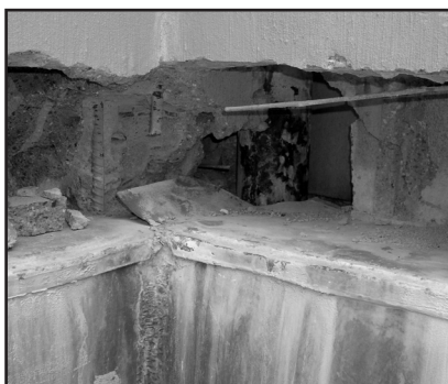
A What's wrong with this picture? Through-wall flashing is not turned up inside the wall, corner laps are insufficient, and reinforcing bars penetrate flashings. The result: multiple points for water entry.
