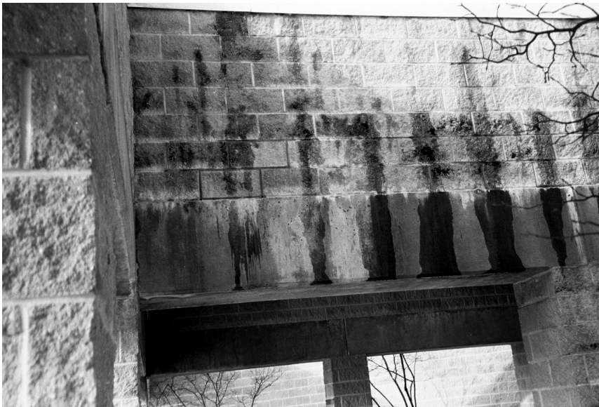
▲ Failure to properly detail and build this concrete block wall left it open to water entry, which led to toxic mold growth. Exterior wythes must be demolished and rebuilt, wasting materials and energy.
