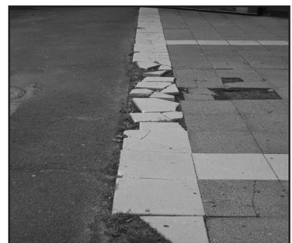
A Design flaws permit water entry and lead to premature breakdown of components. After only a few years of use, this plaza must be ripped up and replaced, wasting energy and resources.
