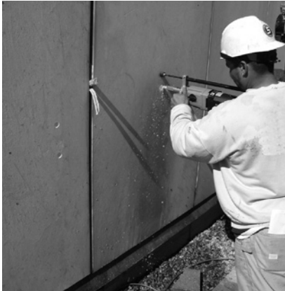
▲ Face-pinning is often used as a safety measure to prevent loose panels from falling.
