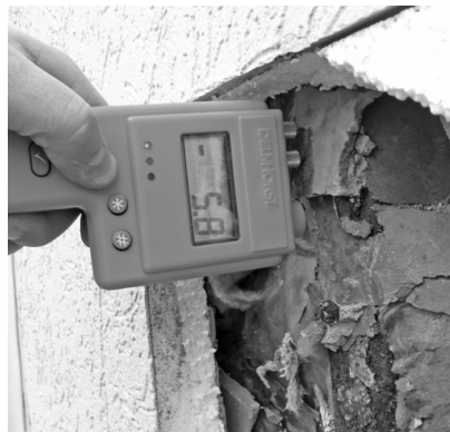
▲ Moisture meters may be used as part of an EIFS failure investigation.
