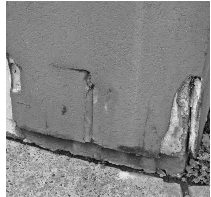
▲ Impact damage that is not repaired promptly provides a pathway for leaks.
