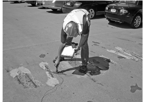
▲ Half-cell potential readings can be used to identify areas of reinforcing steel that are at greatest risk of corrosion.
