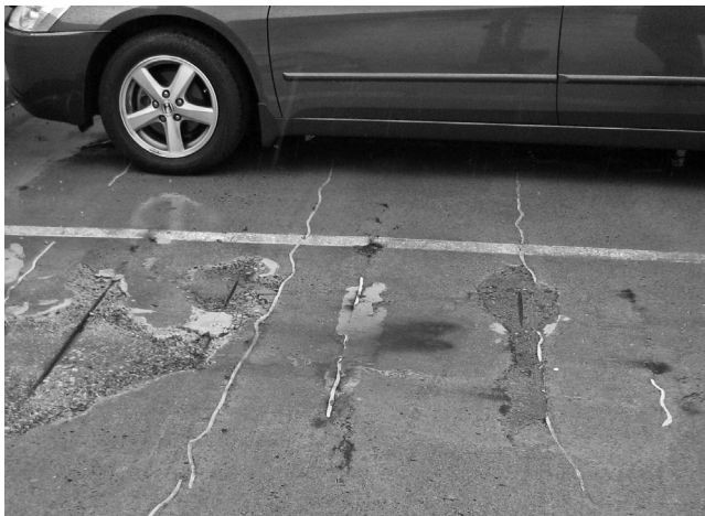
A Corrosion of embedded steel reinforcement is a leading cause of premature deterioration in parking garages.
