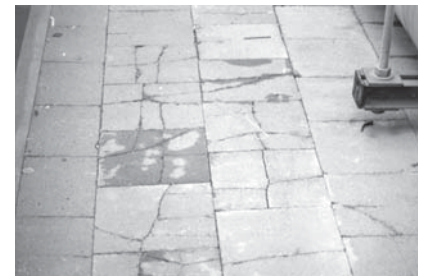
▲ Note cracks in these damaged ballast pavers (in a low slope system).
