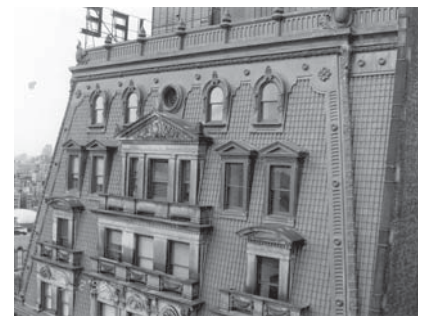
▲ An historic mansard roof (having on each side a steeper lower part and a shallower upper part) with terra cotta tiles.
