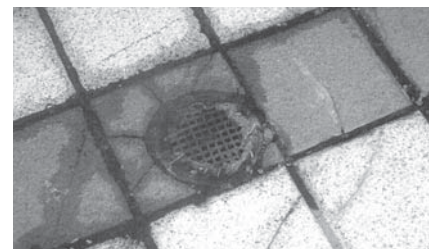
▲ Debris should be cleared of drains to ensure their effectiveness. Note cracks which permit water entry.
