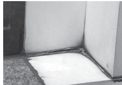
A Cohesive joint failure.
