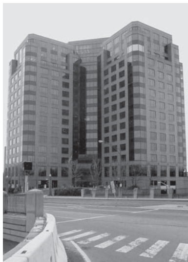
▲ Water infiltration, thermal expansion/contraction, improper construction or substandard materials, structural movement or stress, and age contribute to the inevitable deterioration of building materials over time.
