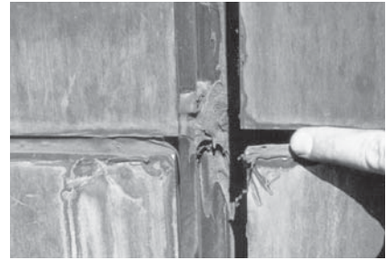
A Sealant failure between aluminum panels.
