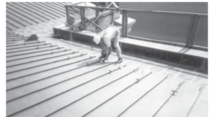
▲ Open seams/solder joint failure are indicators of deterioration in metal systems. Proper care during application of roofing materials is critical to preserving a roof’s useful life.
