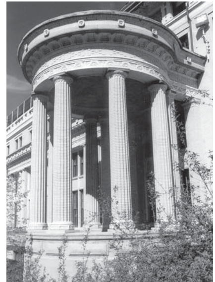
▲ Intricate patterns and decorative elements can present challenges when rehabilitating historic structures.
