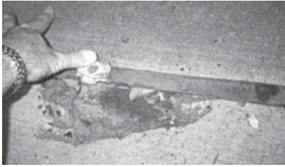
▲ Spalls, laminations that break off due to corrosion of reinforcement/embedded items, are among the indicators of failure in parking structures.
