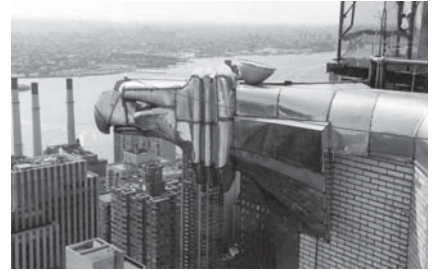
▲ Large, stainless steel replicas of automobile hood ornaments adorn the landmarked Chrysler Building. Over the years, roofing mastic, sealant and other incompatible materials were used to make repairs, all of which exacerbated negative conditions.
