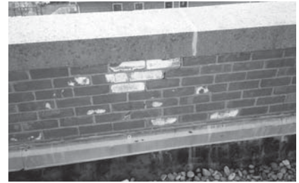
▲ Efflorescence, white stains and/or build-up of white, crystalline structures, is caused by the dissolution and surface deposition of naturally occurring salts.
