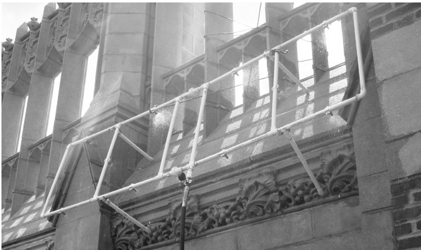
▲ As part of a defect survey, spray rack water tests quantify the extent and location of water penetration.
