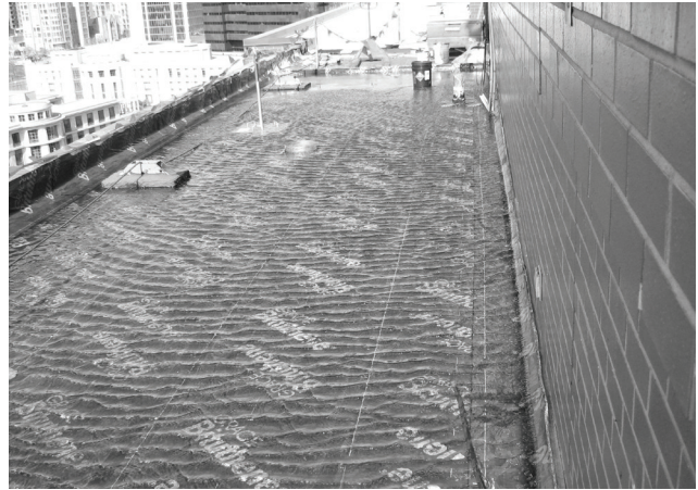
▲ Flooding a newly installed roof membrane to check for leaks is often part of the reroofing process.
