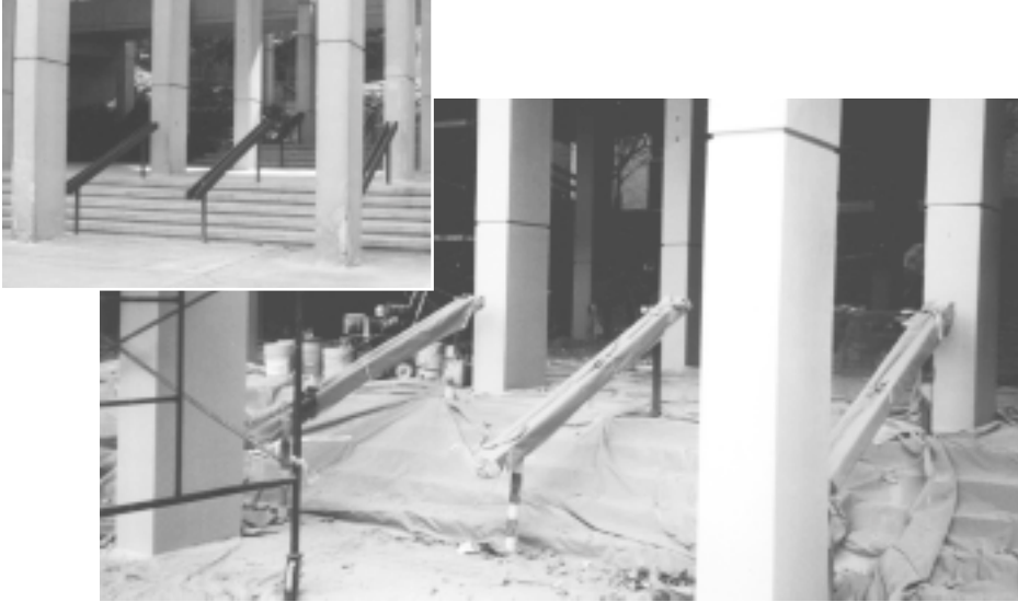
▲ When coupled with proper investigation and repair, coatings can be successfully integrated into a waterproofing project. Not only does this coating improve the water repellency and carbonation retardance of these concrete columns, it enhances their appearance as well. Note the use of cloth coverings to prevent overspray from accidentally damaging surrounding surfaces.
