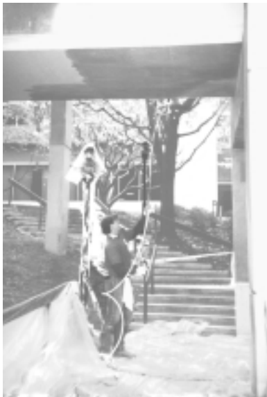
▲ A worker spray-applies a breathable elastomeric coating to a concrete corporate facility.
