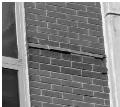
▲ Figure 2a: Brick displacement due to poor flashing design and freeze/thaw cycling.
