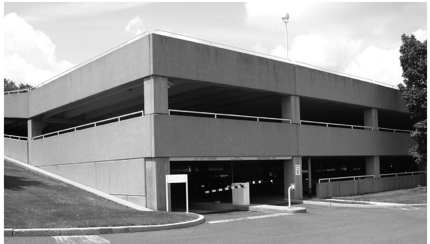
▲ BMW of North America Headquarters in Woodcliff Lake, New Jersey. Garage Rehabilitation.
