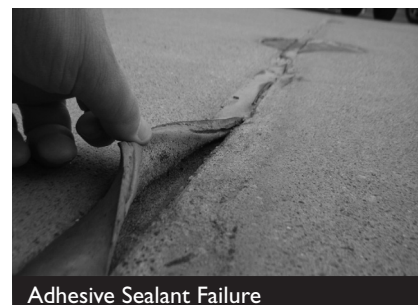
Adhesive Sealant Failure
