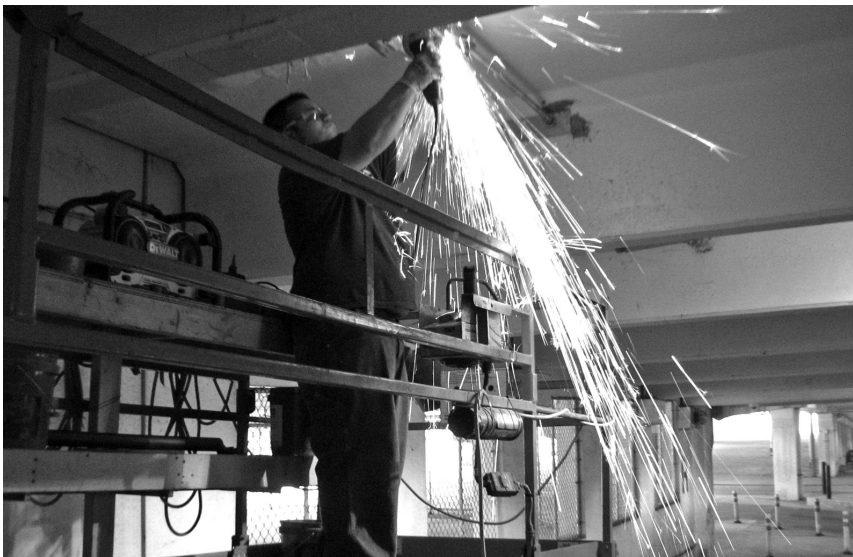
▲ Trimming a chord connection rod as part of a precast concrete garage rehabilitation.
