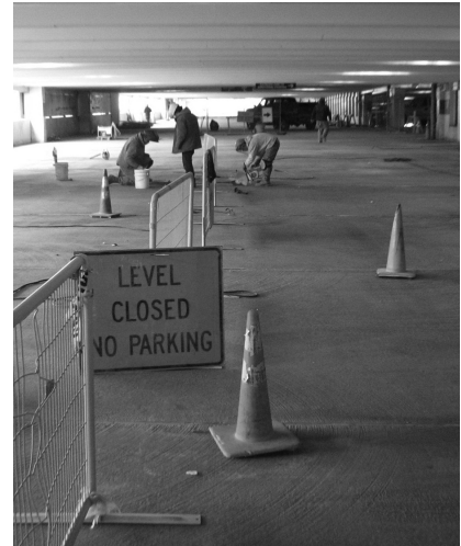
A Coordinate repairs to maximize continuous operation.
