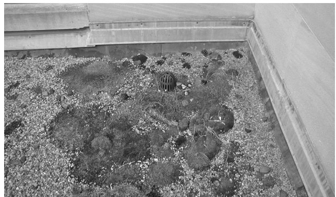
▲ Organic growth and debris on a built-up roof.
