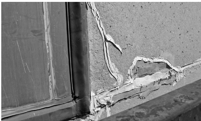
▲ Inappropriate crack repair using surface-applied sealant.
