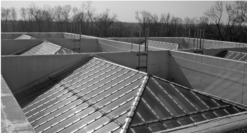
▲ An integral part of the balance of light and mass in many Modernist buildings, skylights are also notorious for leaks, condensation, and poor energy performance.
