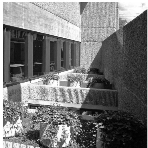
▲ The restoration recreates the original aesthetic, admitting natural light while resolving leaks and improving thermal performance.
