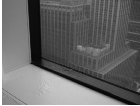
Water pooling at sill.
