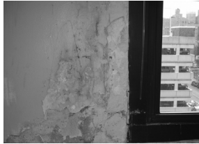
Interior finish damage.
