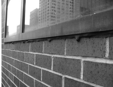
Sealant failure at window exterior.
