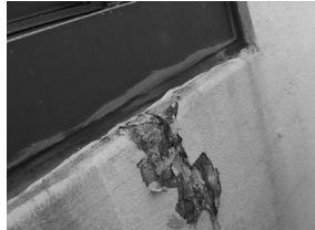
Exterior finish damage.
