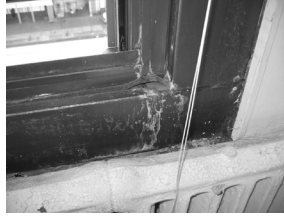
Stains on frame.
