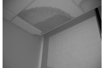
Water intrusion and interior damage.
