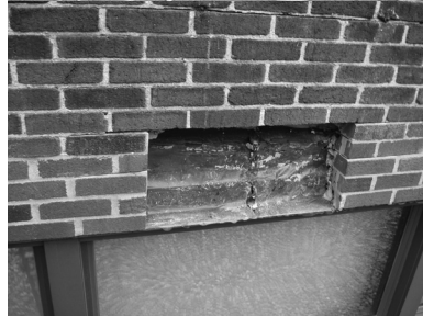
Damaged flashing at window head.
