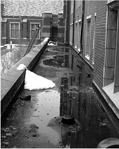
A Ponding water on roof setback.
