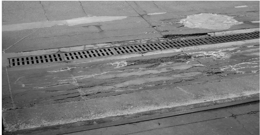
▲ Steel plow blades can cause substantial damage, particularly at drains, joints, and transitions.
