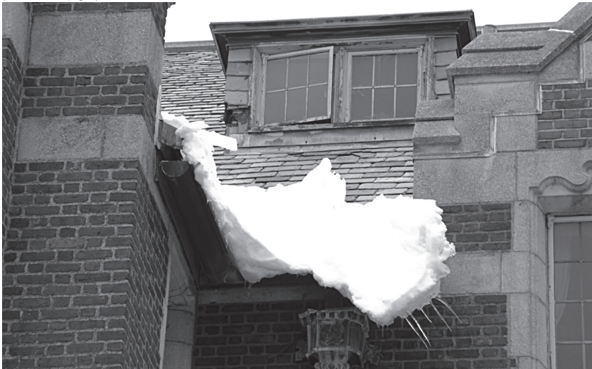
▲ Ice dams pose serious hazards and, over time, lead to roof damage and leaks.
