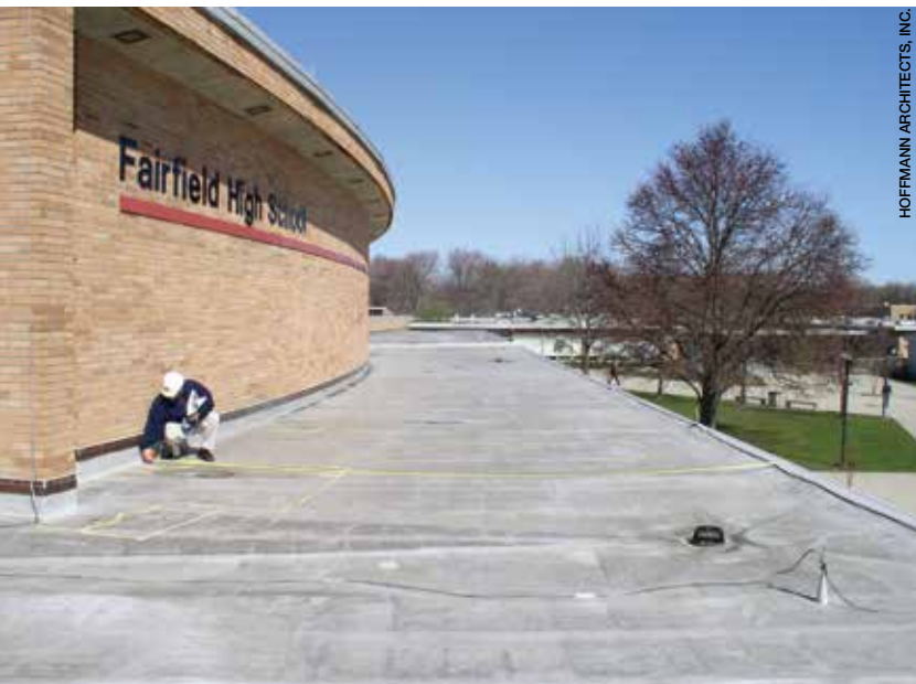
A comprehensive survey of roof conditions at Fairfield, Conn., public schools evaluated roof assemblies and provided condition summary reports and a roof preventive maintenance manual for the town's sixteen schools.
