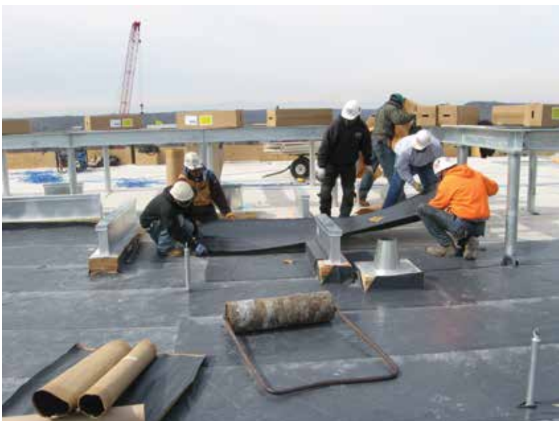
Roof design detailing must account for building-specific needs, such as the presence of many penetrations.
