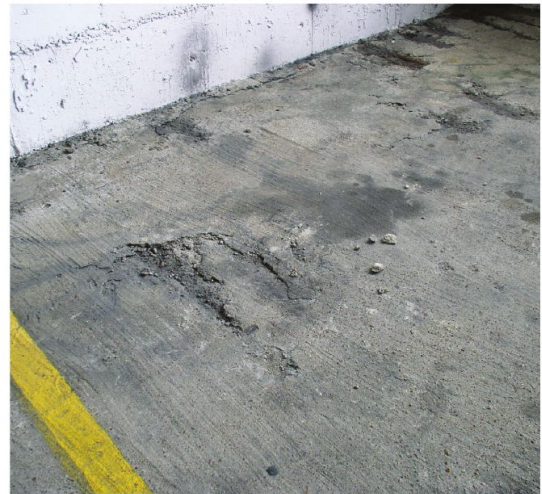
Surface spalling on a concrete parking deck due to corrosion of embedded steel reinforcement.
