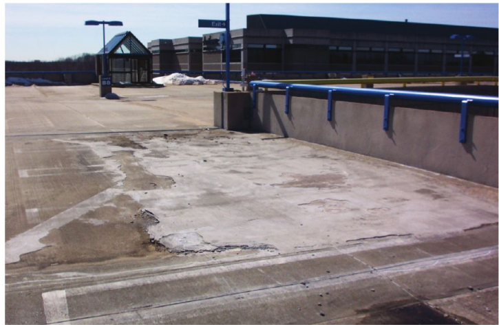
Disintegrated concrete overlay on top deck of precast concrete parking structure. Concrete overlays can easily chip and spall when the edges are feathered out instead of squared off.
