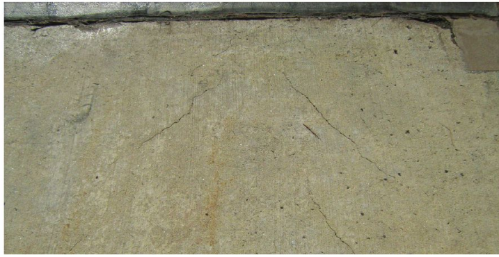
Chevron cracks, such as the parallel diagonal fissures that are shown above in a repeating 'V' pattern, are typically caused by shear stress.
