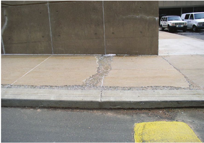
The photo above shows a crumbling concrete sidewalk due to freeze-thaw cycling and applied de-icing compounds.
