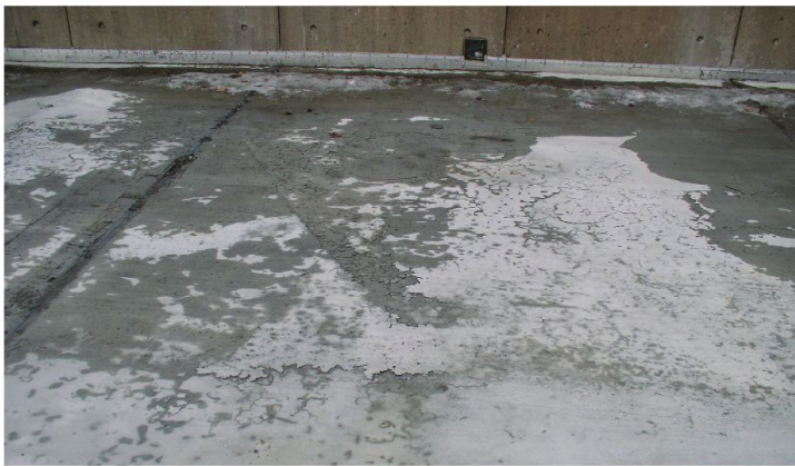
Concrete that is often saturated with water and exposed to freeze-thaw cycles may experience scaling, or flaking and peeling of the surface.
